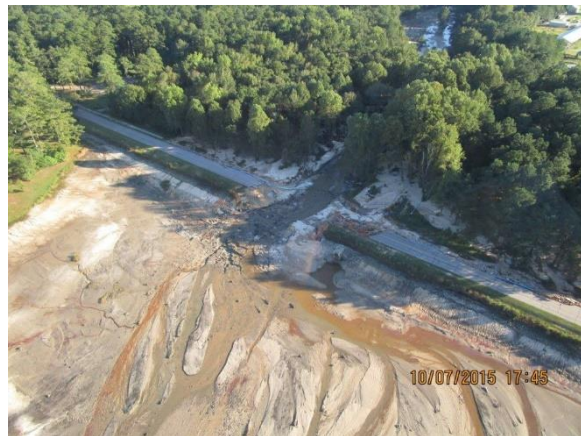
Semmes Lake Dam failure
