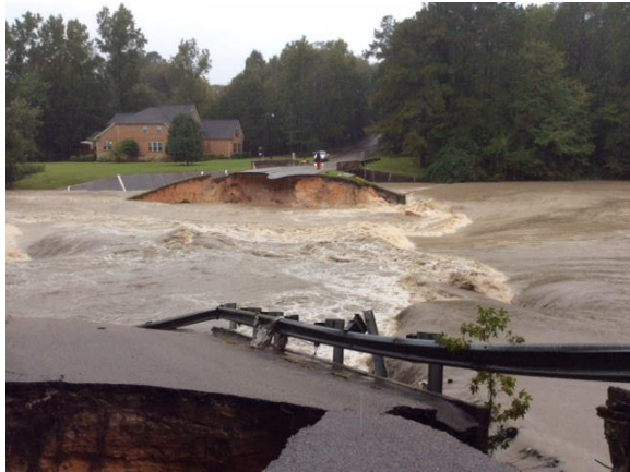
Carys Lake Dam failure
