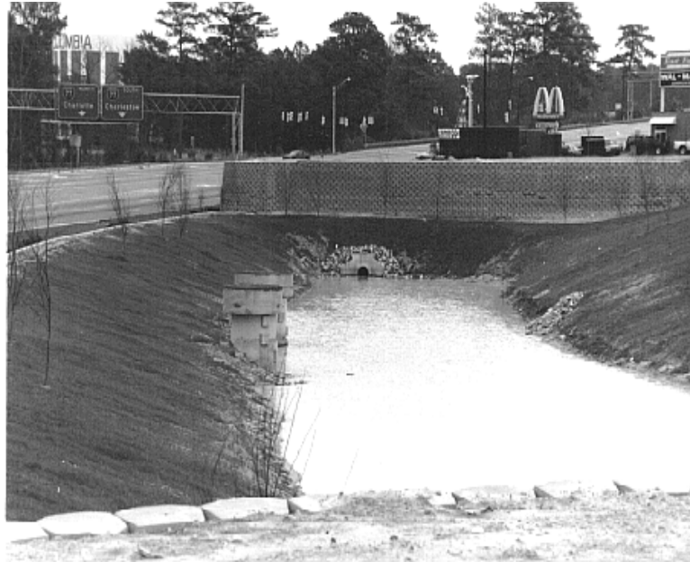
Stormwater detention basin serving the Forest Dr. Wal Mart complex
